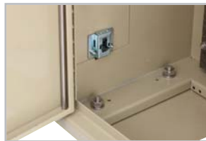
cable entry door (inside)
